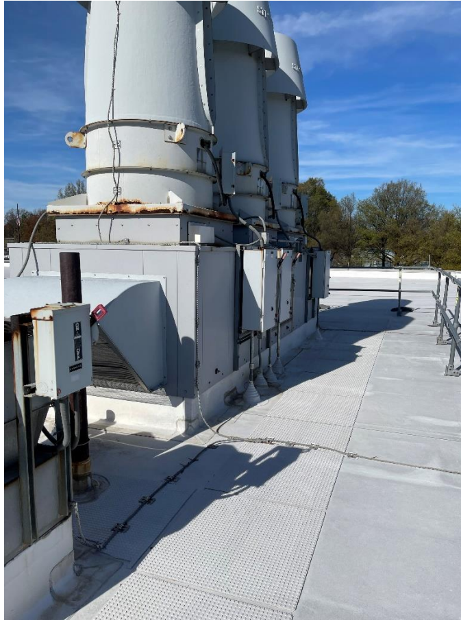
Photo # 26: Equipment on the Mechanical Building
