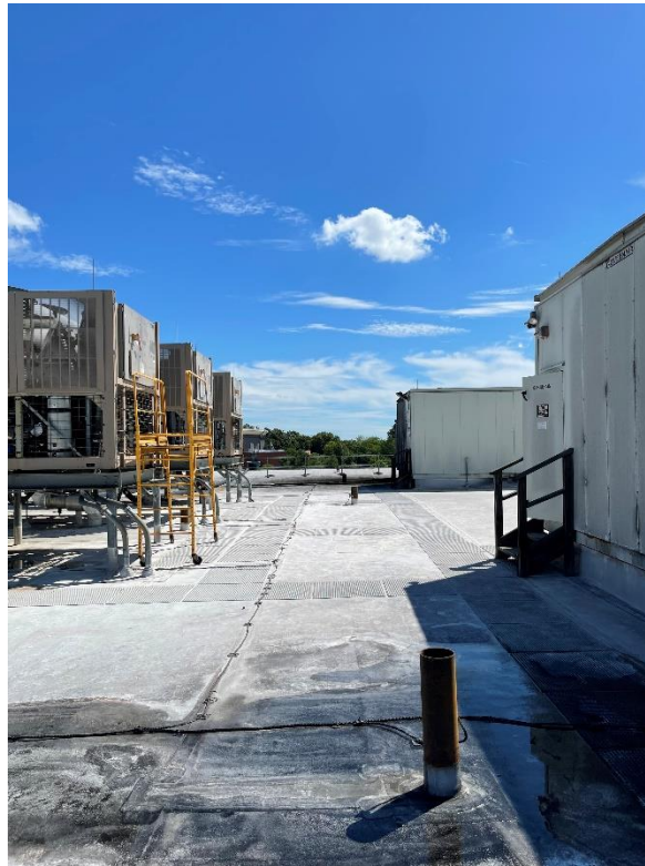
Photo #13: Looking towards the space between Chiller and AHU units
