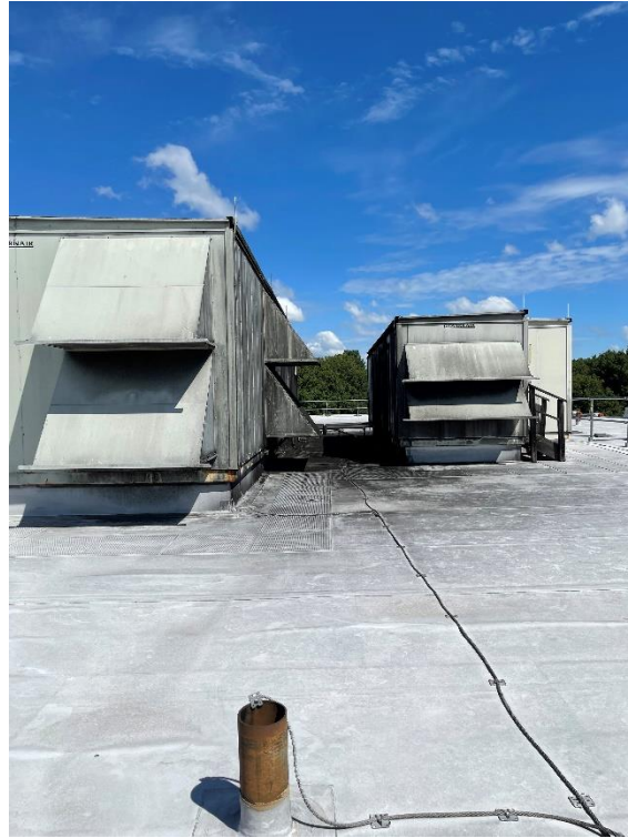
Photo #8: Looking towards AHU-2 and AHU-5
