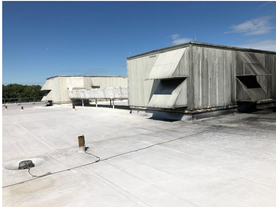
Photo #6: Looking towards AHU-2
