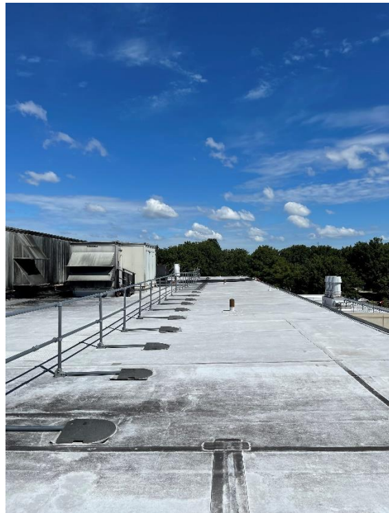
Photo #10: Looking towards Chiller and AHU-5
