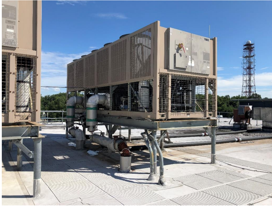
Photo #14: Looking towards the Chiller unit
