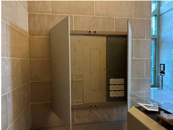
Photo 08: electric panels in Coatroom 0015, to be reconfigured.
