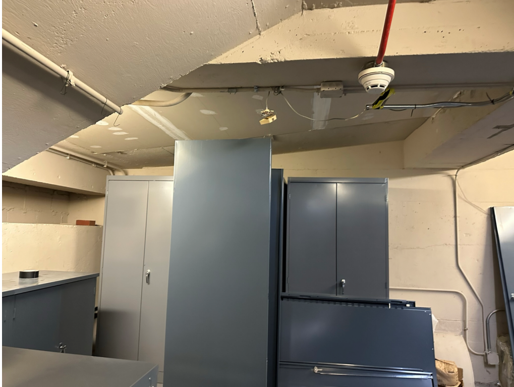
Photo 11: in Mezzanine, concrete beams & deck above; sloped concrete below stairs; GWB ceiling area at steel deck infill.
