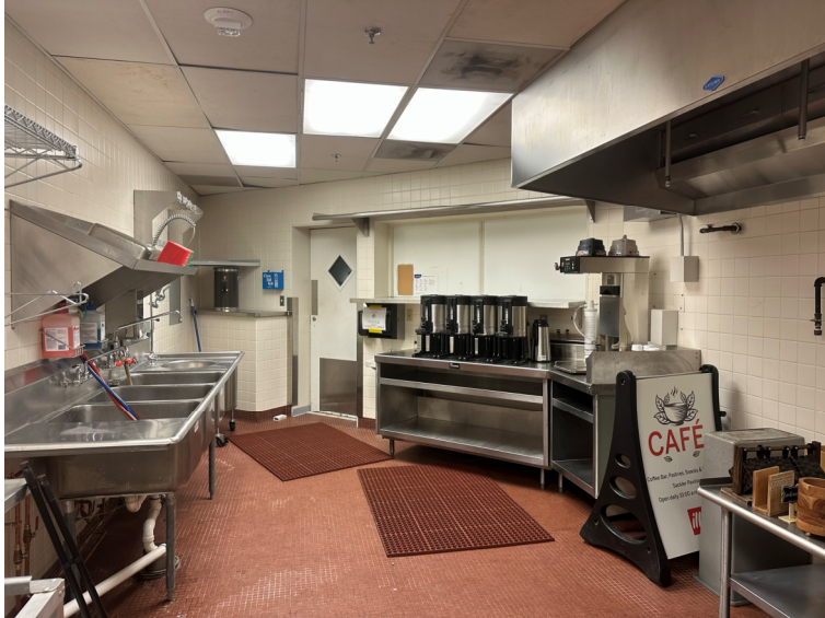
Photo 16: Kitchen 2020: ETR 3-compartment sink; range has been removed and gas capped; see new layout for new equipment.
