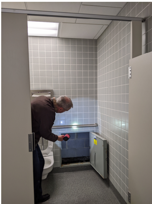
Photo 15: Men's room in front of chase will that will hold new piping to riser. Wall is 4x4 ceramic tile on GWB and steel studs. Access panel pictured.
