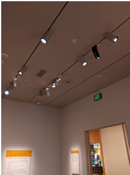
Photo 12: Gallery 1075, showing ceiling type and devices to be removed and reinstalled. Piping will run above this ceiling between Gallery 0012 and Mezzanine 0014.
