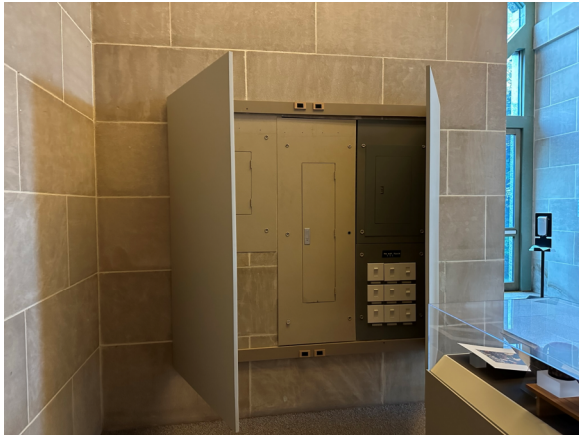
Photo 08: electric panels in Coatroom 0015, to be reconfigured.
