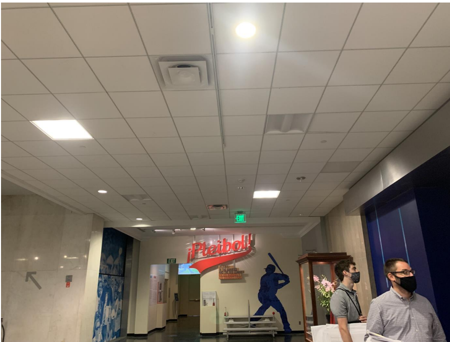
Figure 11: Ceiling in public space outside of Lounge 2E. R&R ceiling between Lounge and Toilet Rooms to install piping (see Drawings.)
