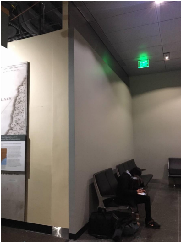
Figure 15: New screen wall in front of Gift Shop is painted gwb on steel studs. (3/17/22)
