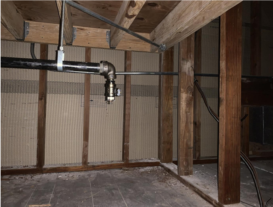
Figure 10: Concealed space below Lower Mezzanine. Note expanded metal mesh on walls of Collections Storage.
