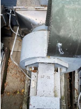
EF-11 – Serves room 1109 fume hood. Located on the rooftop of stairwell 1006. Switch operated in the space. Starter location 1096ER / Breaker Panel HDP1C.
