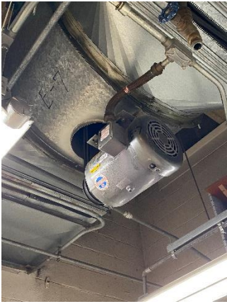
EF-9 – Serves the projection booth for the lecture hall 2 nd level. Located in the doghouse of stairwell 1007. Starter location 1049ER.
