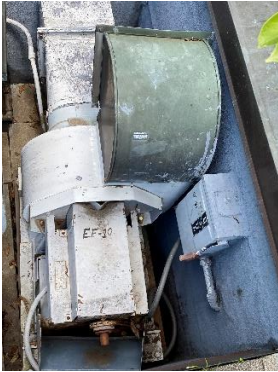
EF-10 – Serves room 1109 fume hood. Located on the rooftop of stairwell 1006. Switch operated in the space. Starter location 1118ER / Breaker Panel HDP1B.
