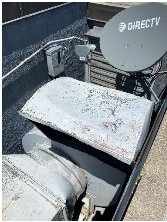
EF-5A – Serves the mechanical room and is located on the roof of stairwell 1003.
