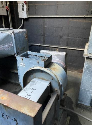
EF-10 – Serves 1113 photo lab on the 1 st level African art. Located on the rooftop of stairwell 1006. Starter location 1118ER / Breaker Panel HDP1B.
