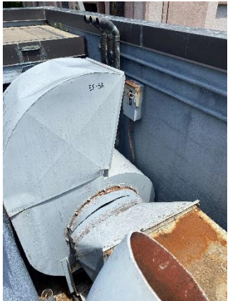
EF-6 – Serves the loading dock and is located in the loading dock. Starter location 1049ER / Breaker Panel HDP1A.
