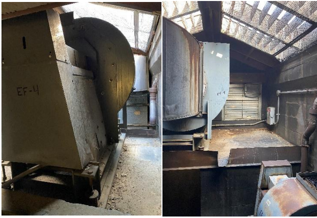
EF-5 – Serves the mechanical room and is located on the roof of stairwell 1002.
